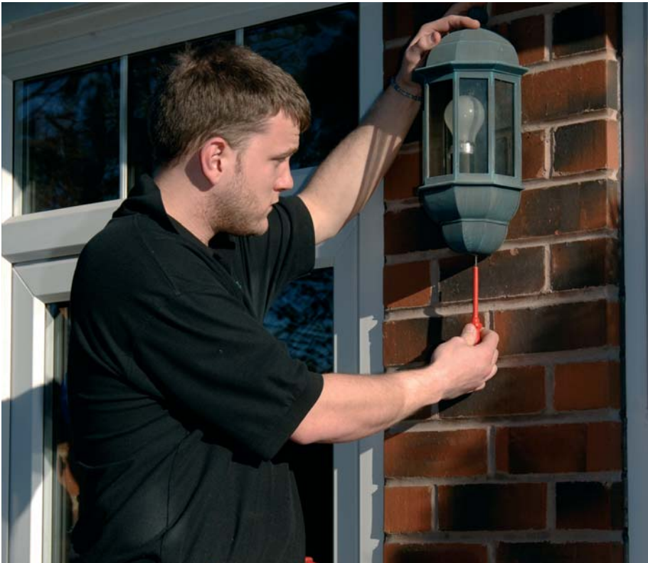
Outside Lighting subject to Part P
