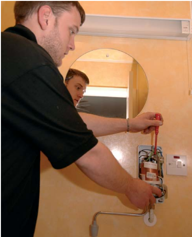
Electrical work in Bathrooms. High risk of electrocution if not installed correctly
