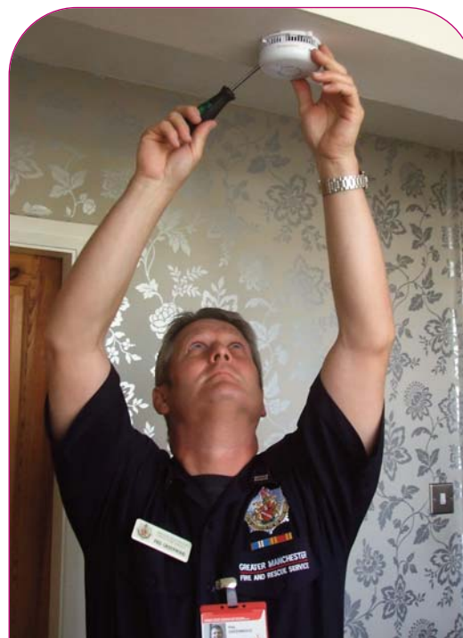
Greater Manchester Fire and Rescue Service will install smoke alarms for FREE as part of their Home Fire Risk Assessments
